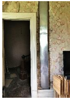
Heat ducts in the parlor.
